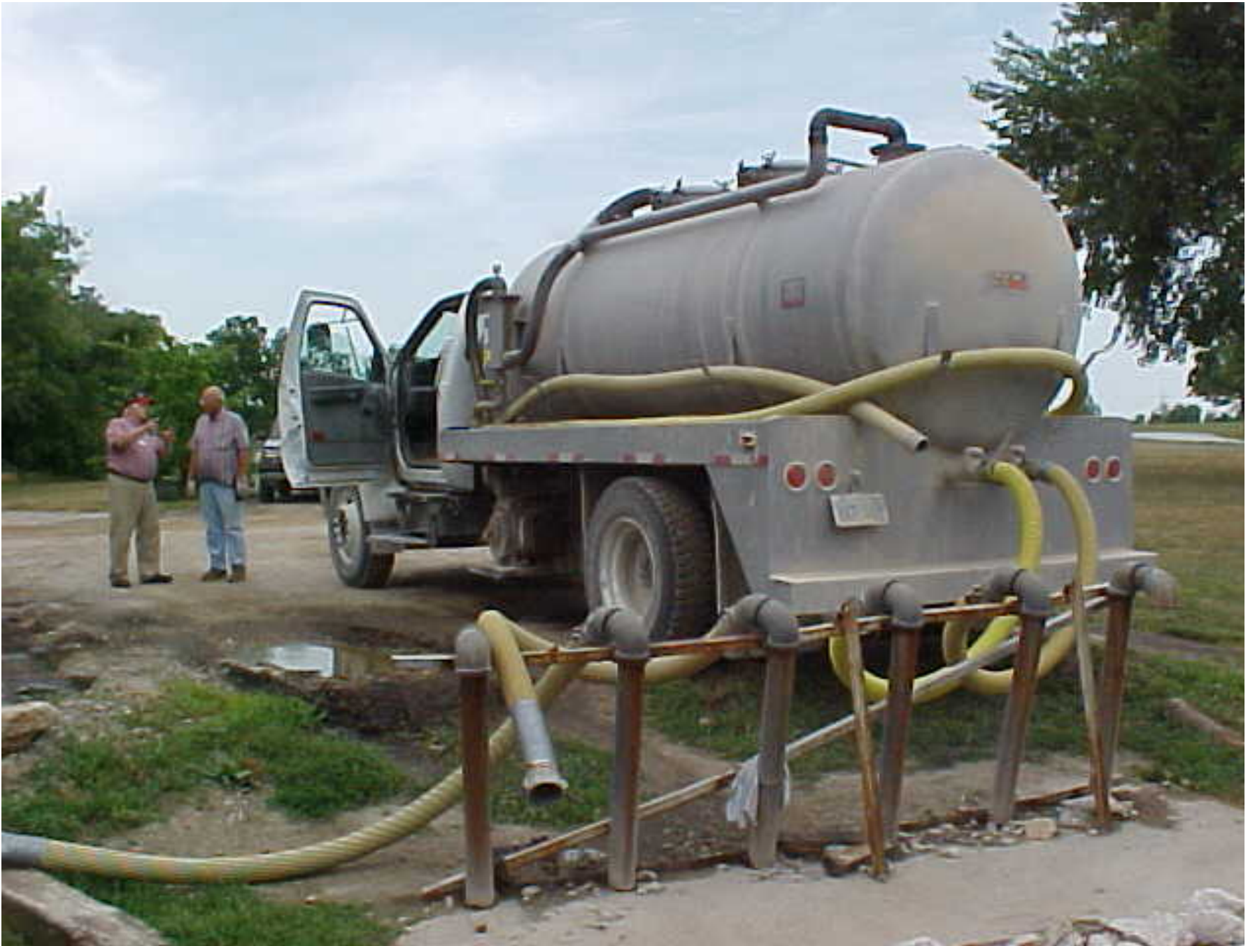
SEWER PUMP TANK AND PUMP STATION
