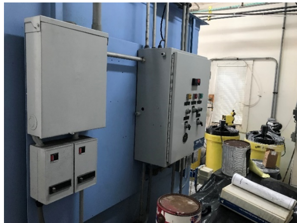
Photo 1: Water Treatment Package Plant Exterior
