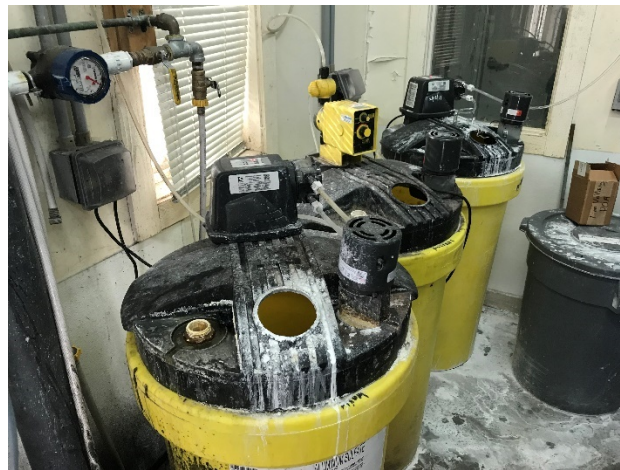
Photo 3: Chemical Feed Units
