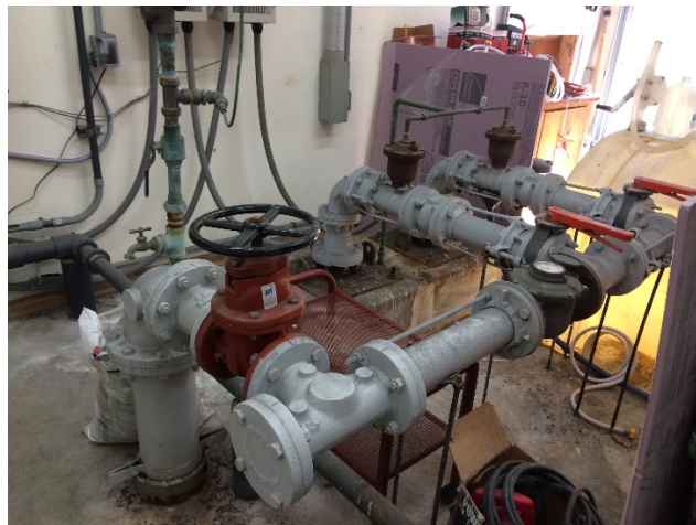
Photo 4: Piping to Clearwell
